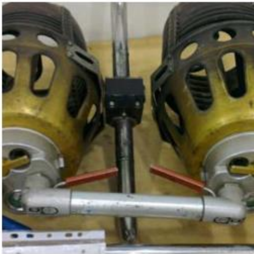
Fig 1. Double Stratus Burner Unit Note failed hanger on the right.
