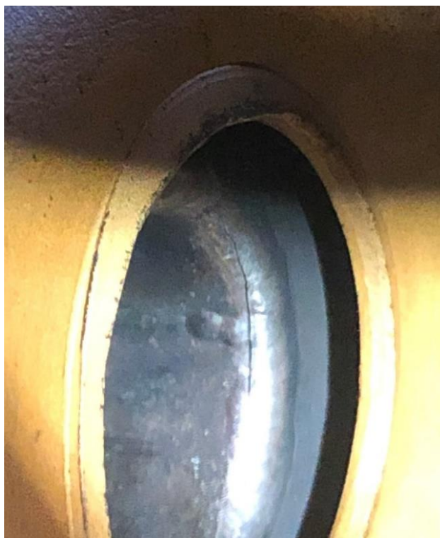
Fig 1. Hanger with Weld Crack.
